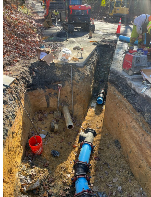
Installation of a replacement waterline in Town Creek as part of the Phase 2 replacement project.
