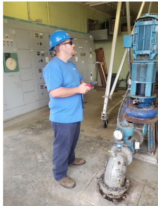
MetCom staff are trained in all aspects of facility maintenance. From rebuilding pumps to making electrical repairs, MetCom employees exhibit a dynamic skill set.
