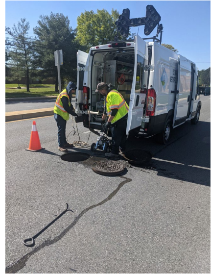
The Collections' Department Sewer Inspection crew utilizing remote viewing technology to pinpoint failing sections of pipe and identify blockages.
