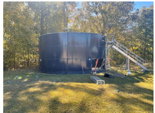
After 30 years in service, the Wicomico Shores WWTP sludge holding tank was taken offline for an inspection, reconditioning and seam recaulking. The sealant is used to ensure that the tank is liquid tight.
