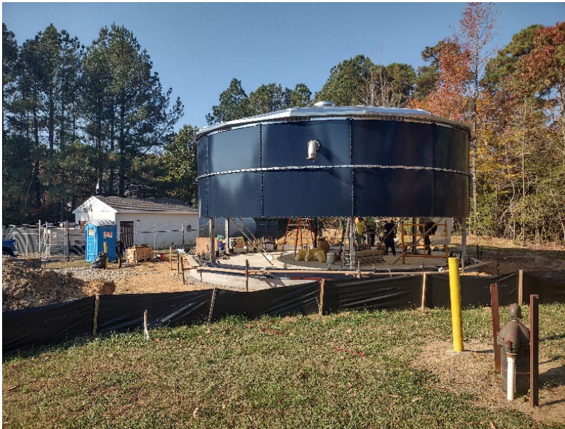
Wicomico Shores Wastewater Treatment Facility sludge holding tank.
