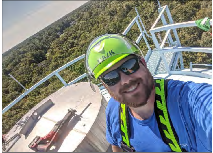
Maintenance work is hard, but it can be fun too. Work on our water towers and communication equipment is ongoing and constant.
