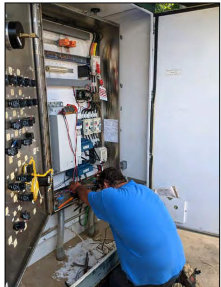
Staff continually works on facilities to keep everything operational. Here a mechanic rewires a faulty control panel.
