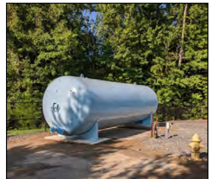
Newly installed hydro pneumatic water tank at the Wild Goose Crest water station.
