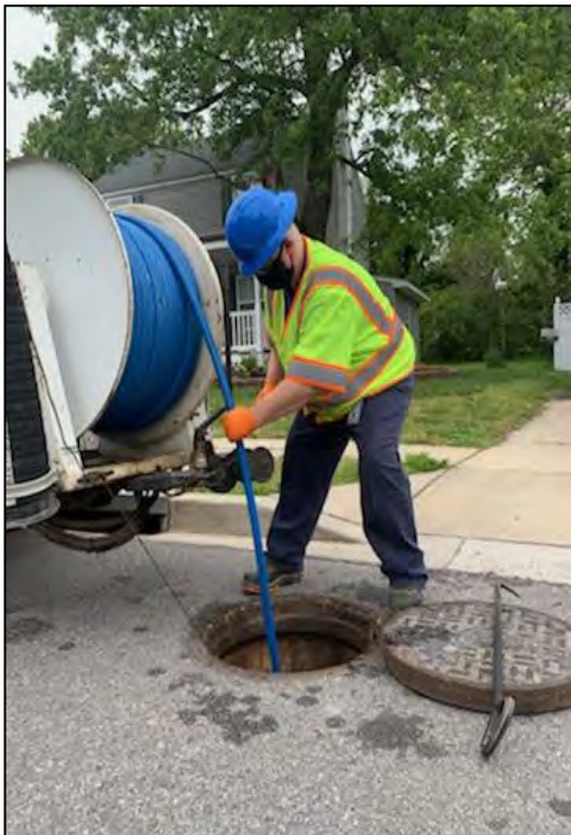
Clearing and cleaning sanitary sewer lines is ongoing, even in the midst of a pandemic.
