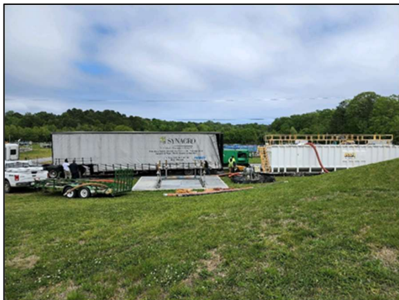
Work on the digester at the Marlay-Taylor Facility consists of draining and dewatering the digester tanks.
