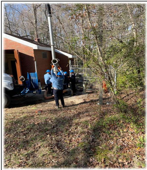
Staff is always working to improve our system. Here, the maintenance staff is cleaning the wetwell at one of our pumping stations.
